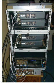
Equipment setup in tower
