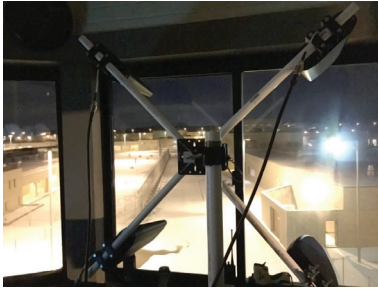
Directional antenna setup in tower pointing toward targeted area
